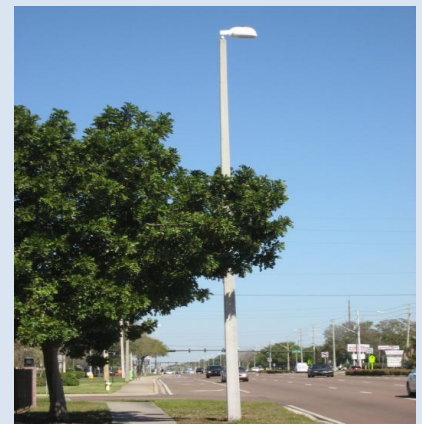
Existing mongoose street light
