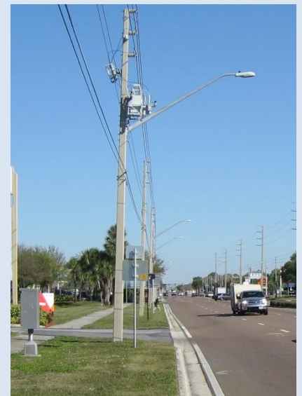
Existing cobra street light
